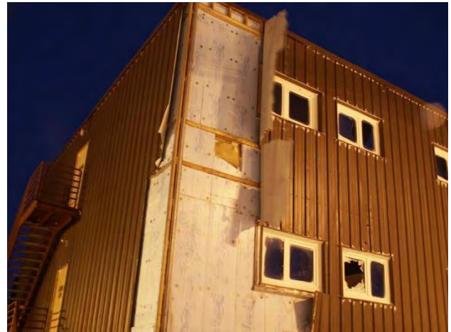
Dormitory With Storm Damaged Siding.
