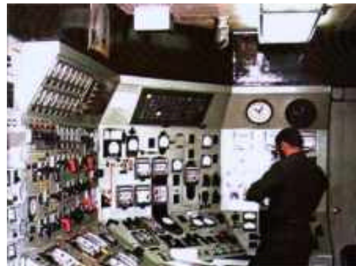
NNPU Control Panel
