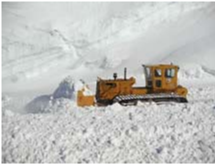
An older model Challenger D-8 tractor clears snow near McMurdo Station. The bulldozers have a wider track than newer models, making them more suitable for such work. Photo courtesy of Larry Cook
